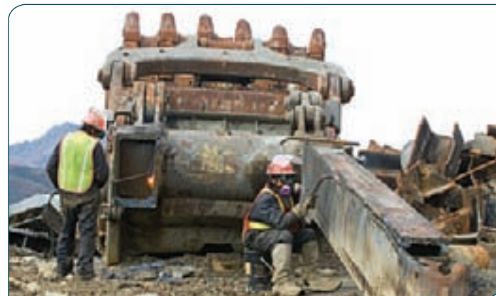
RRDC employees cut abandoned machinery down to scrap metal for removal from the Faro Mine complex.
