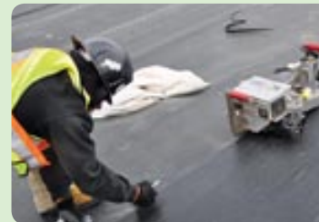
This machine, similar to a sewing machine, melts overlapping edges of liner together. The liner installation crew ensured the liner was properly sealed to protect the waste rock from being exposed to the elements.
