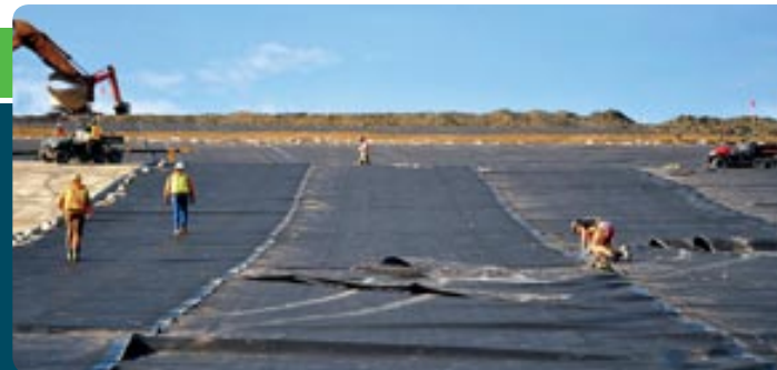
Once installed, the liner covered a surface of about 275,000 m 2 of the Grum Sulphide Cell waste rock. Photo: Government of Yukon
