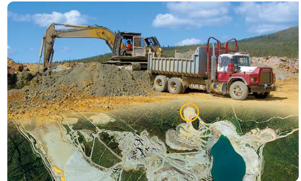
Early remediation this summer included moving waste rock from the Northwest Dump away from Guardhouse Creek to control contamination.
